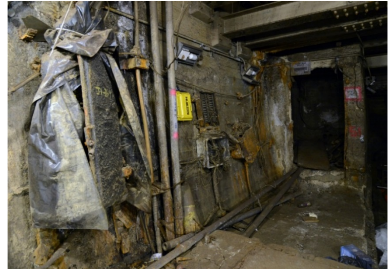
NY MTA—Montague Street Tunnel corrosion after flooding with 20 feet of salt water.
