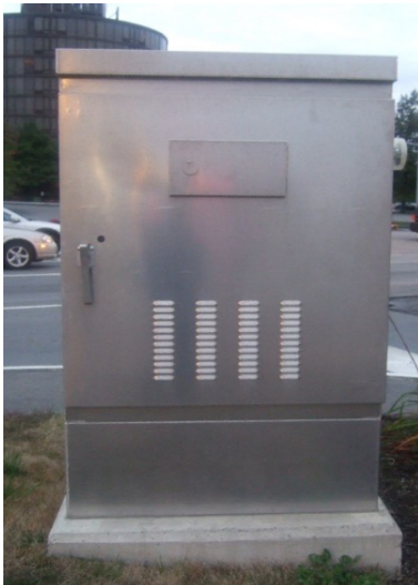
Typical Existing Cabinet
